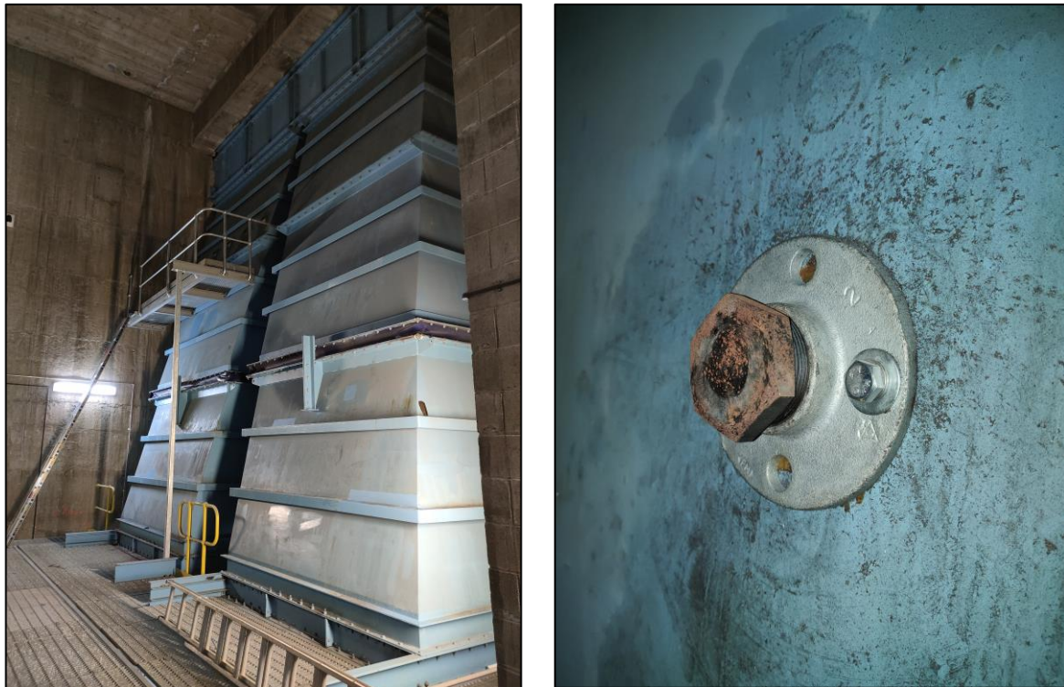
Figure 1: Inside ventilation facility (left) & sampling port (right) e
